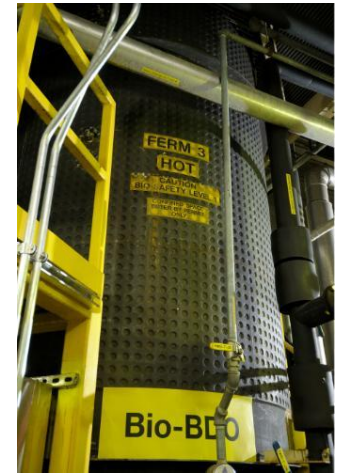
Tate and Lyle facility in Decatur, Illinois. A 3,000 liter fermentation pilot plant. Commercial production of Bio-BDO in 2012.
