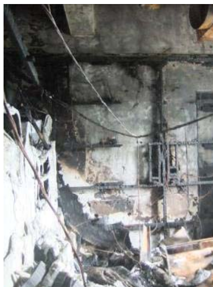
Extensively use corrosive acids causing electrical short circuit and fire accidents
